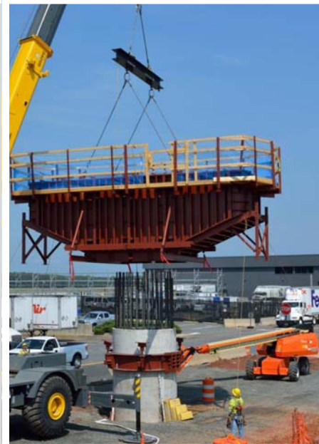
Pier construction in the airport's cargo area. Photo courtesy of Capital Rail Constructors.
