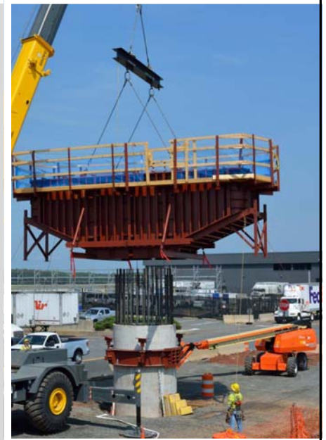
Pier construction in the airport's cargo area. Photo courtesy of Capital Rail Constructors.
