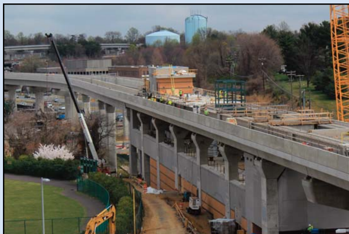
FROM HIGH ABOVE THE TYSONS EAST STATION: Work continues on the Tysons East Metrorail Station. Photo by Chuck Samuelson, Dulles Corridor Metrorail Project
