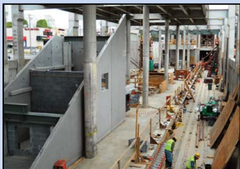
WHAT YOU CAN'T SEE FROM ROUTE 7: The platform, concrete columns, trackway invert and barrier walls are complete for the future Tysons Central 7 Station near SAIC. Photo by Stephen Barna, Dulles Corridor Metrorail Project
