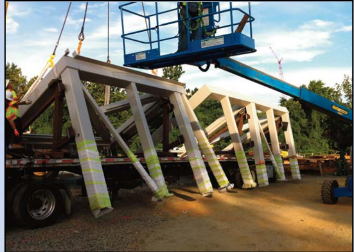
GETTING READY: Components for the pedestrian bridge at McLean Station are already on-site along Colshire Drive. Photo by Dulles Transit Partners
