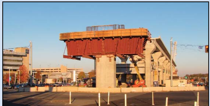
TYSONS WEST: Work continues at the site of the future Tysons West Metrorail Station near Spring Hill Road at Route 7. Photo by Chuck Samuelson, Dulles Corridor Metrorail Project
