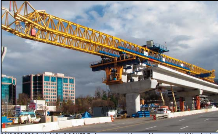
BRIDGES FOR RAIL ALONG ROUTE 7: Crews are making rapid progress building bridges for the Silver Line. Photo by Chuck Samuelson, Dulles Corridor Metrorail Project
