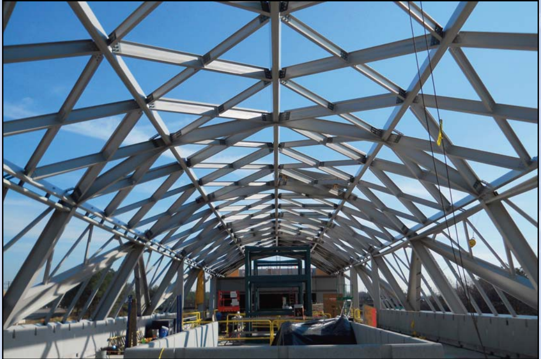
INTO THE SKY AT WIEHLE: Dulles Metrorail crews erect the structural steel canopy on the mezzanine at the Wiehle Avenue Station under construction in the median of the Dulles Airport Access Highway/Dulles Toll Road corridor. Photo by Stephen Barna, Dulles Corridor Metrorail Project
