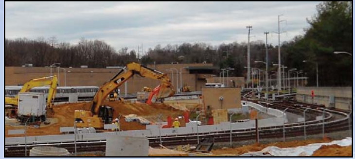
PROGRESS AT THE WEST FALLS CHURCH YARD: Crews complete jack-and-bore crossings for the Service and Inspection building. Photo by Stephen Barna, Dulles Corridor Metrorail Project
