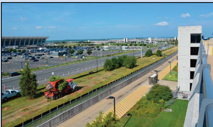
Trees removed from the Dulles Station site will be replanted in other locations at the airport. Photo by Capital Rail Constructors
