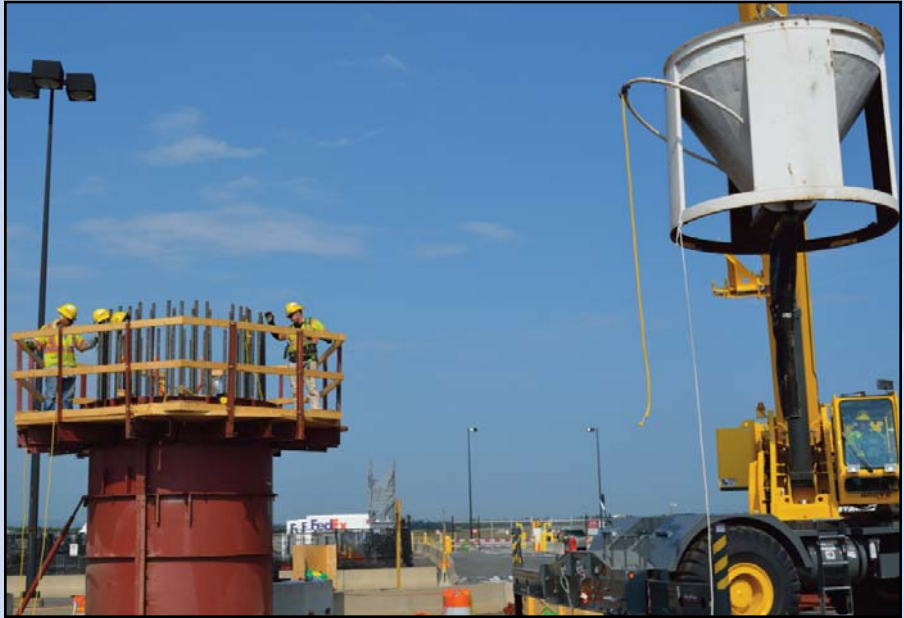
Crews prepare to pour concrete into an aerial guideway column. Photo by Capital Rail Constructors
