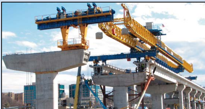
HIGH IN THE SKY: Aerial truss continues to raise segments of bridges into the air near Route 7 and Tyco Road. Photo by Chuck Samuelson, Dulles Corridor Metrorail Project
