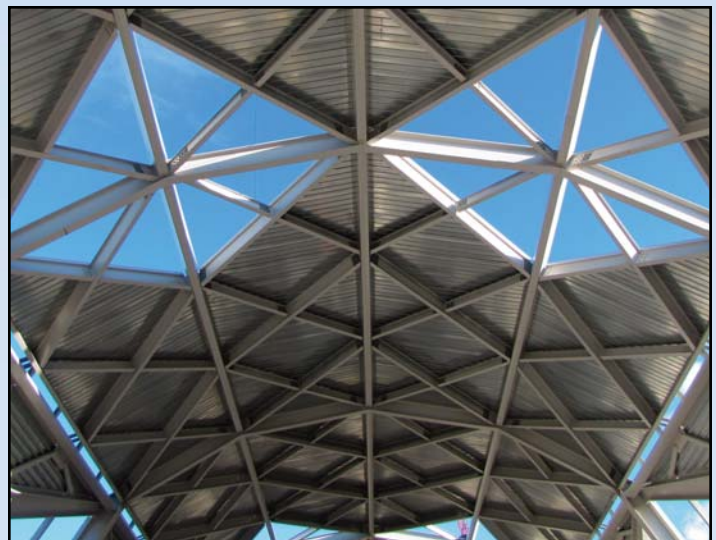
CANOPY AT WIEHLE: The canopy is very visible at the Wiehle Avenue Metrorail Station. Construction of this station is the most advanced of all five stations. Photo by Chuck Samuelson, Dulles Corridor Metrorail Project
