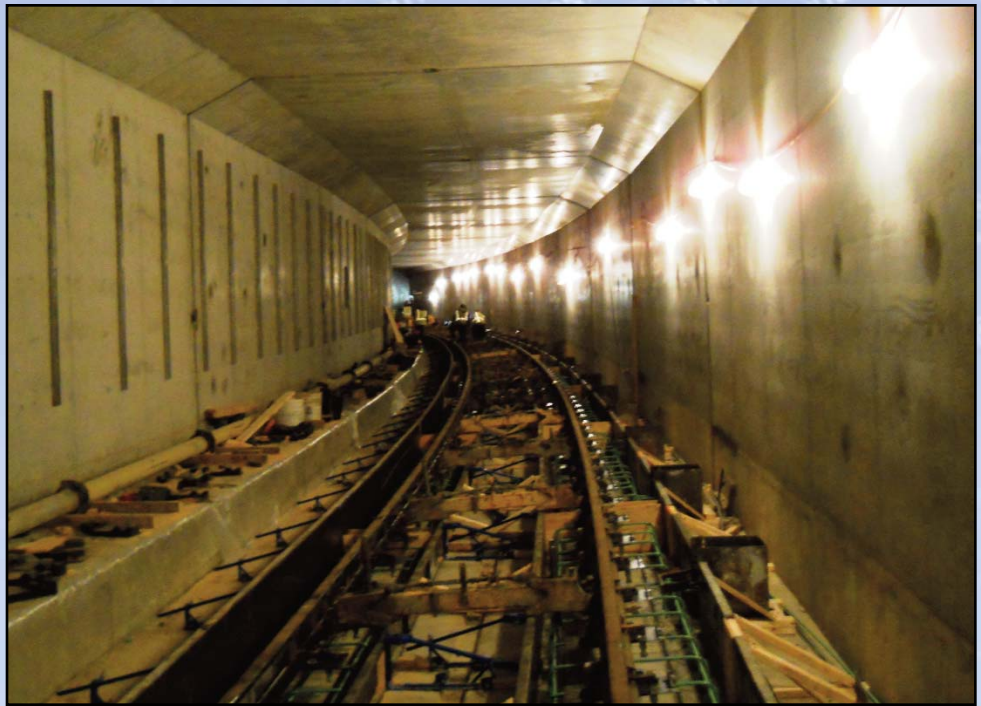
INBOUND TYSONS CUT-AND-COVER TUNNEL: Rails are being set in this portion of the tunnel under Route 7 just east of Route 123. Photo by Stephen Barna, Dulles Corridor Metrorail Project
