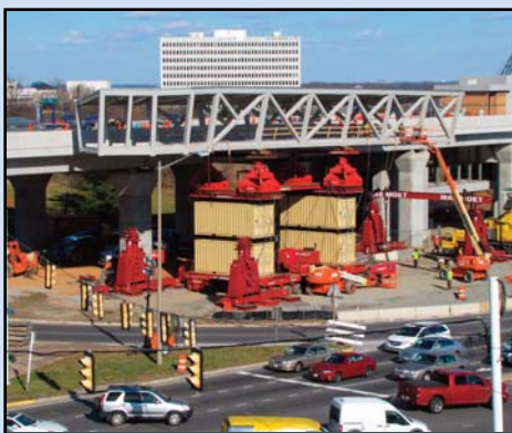
READY TO GO UP: Crews prepare for placement of pedestrian bridge segments at the Tysons Corner Station. Photo by Chuck Samuelson, Dulles Corridor Metrorail Project
