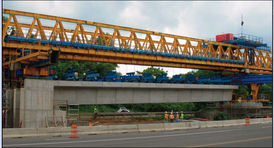
The truss located on the Dulles Connector Road is now in action as it lifts the segments to build the aerial guideway tracks. Photo by Stephen Barna, Dulles Corridor Metrorail Project
