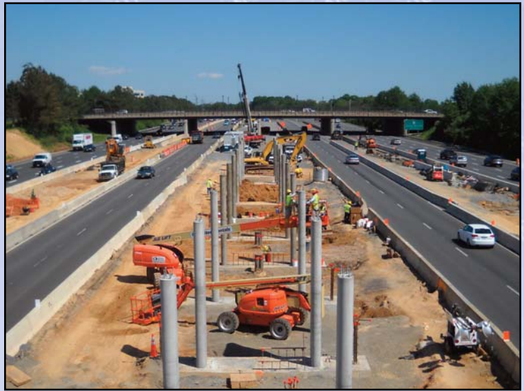
Construction of the Wiehle Avenue Station in the median of the Dulles Toll Road and Dulles International Airport Access Highway. Photo by John Odorisio
