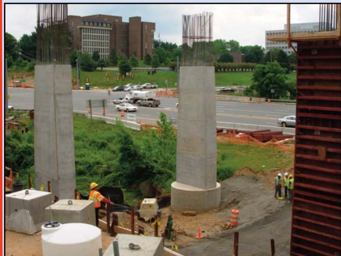
Tysons East Station construction progressing on Route 123 near the Colshire Drive intersection. Photo by Stephen Barna, Dulles Corridor Metrorail Project
