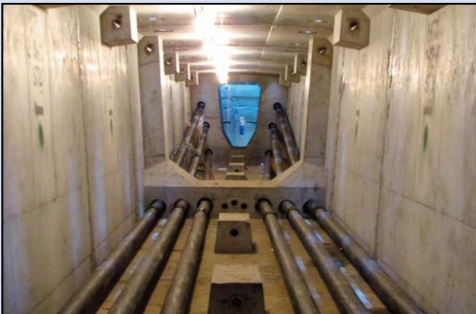
Inside the connected segments being built as part of the aerial guideway. Photo by Dulles Corridor Metrorail Project
