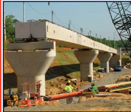
Aerial guideway construction starting near the I-66/Dulles Connector Road interchange. Photo by Dulles Corridor Metrorail Project
