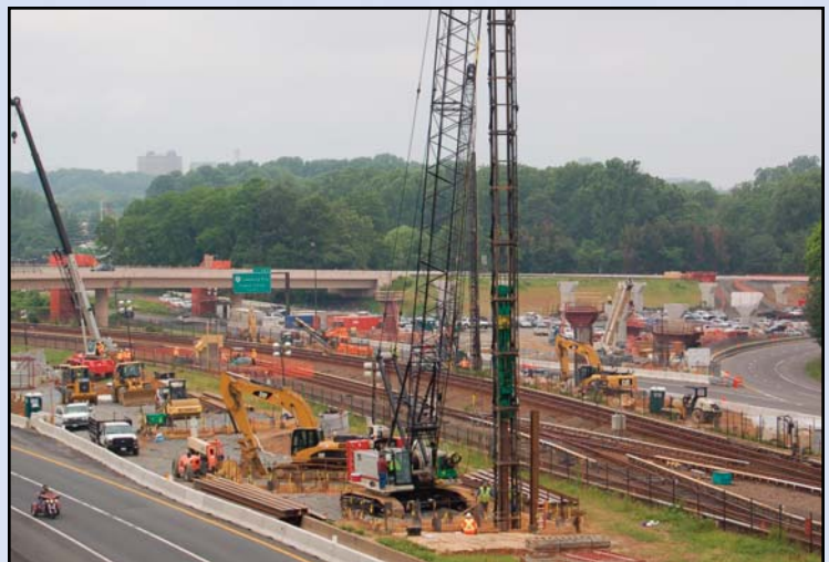
Construction at the I-66/Dulles Connector Road interchange, where the new line will merge with the existing Orange Line. Photo by Dulles Corridor Metrorail Project
