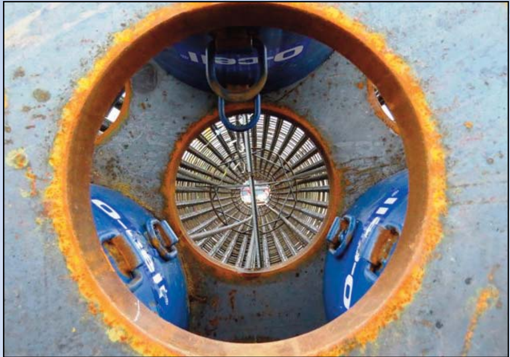
FROM THE BOTTOM DOWN BELOW AT DULLES: This photo from the bottom-up of a drilled shaft foundation rebar cage shows the three Osterberg Cell piston and pressure chambers used for testing the foundation design for the future elevated guideway for tracks at Dulles Airport. Photo by Chuck Samuelson, Dulles Corridor Metrorail Project
