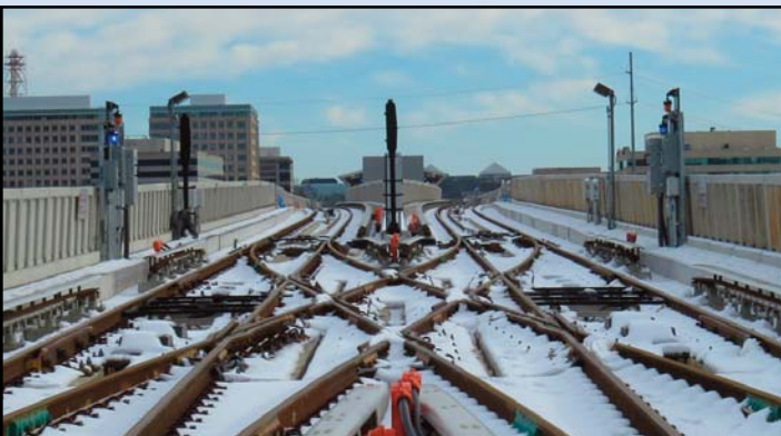
WINTERTIME: The recent snow atop the tracks in the median of Route 7. Photo by Chuck Samuelson, Dulles Corridor Metrorail Project
