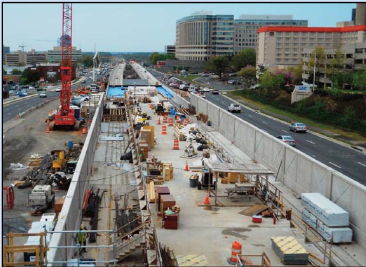
VIEW FROM ABOVE ROUTE 7: Looking west from the mezzanine deck at the top of the escalator opening at the Tysons Central 7 Station, aerial guideway for rail is visible as it winds toward the Tysons West Station. At the station, the concrete platform deck and barrier walls are complete and the invert slabs in the inbound and outbound track ways are almost complete. Photo by Stephen Barna, Dulles Corridor Metrorail Project
