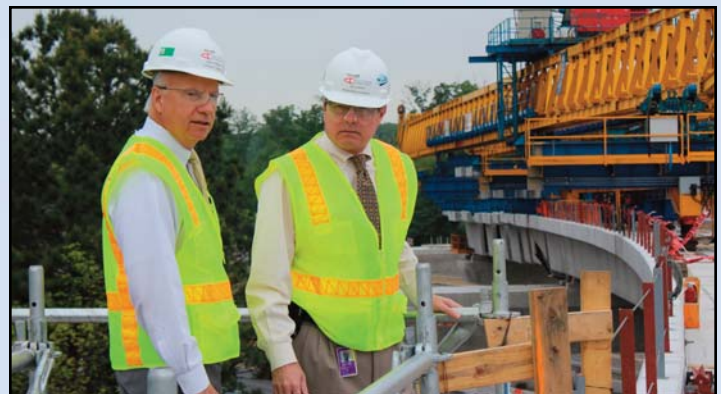
SMILE!: Project Director Sam Carnaggio, left, and Kevin Volbrecht, Deputy Director for Construction, atop the guideway from Route 7 to the median of the Dulles Access Highway. Photo by Chuck Samuelson, Dulles Corridor Metrorail Project
