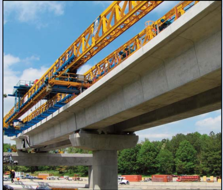
BUILDING FINAL SPANS: The large horizontal crane is now being used to construct the bridge spans across the Dulles Toll Road to carry rail bridges from Route 7 to the median of the Dulles Toll Road. Photo by Chuck Samuelson, Dulles Corridor Metrorail Project
