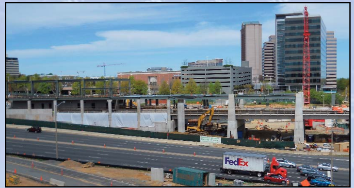
NOW: The Tysons Central 123 Station is now very visible as construction proceeds at Route 123 and Tysons Boulevard. Photo by Stephen Barna, Dulles Corridor Metrorail Project
