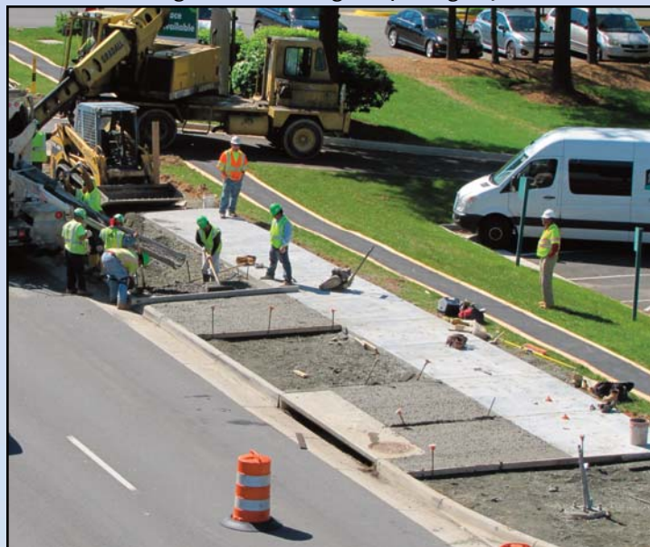
EVIDENCE OF SIDEWALKS: Dulles Rail crews are continuing to build sidewalks and create spaces for plantings and street lights along Route 7. The light poles will later be installed by Dominion Virginia Power. Photo by Chuck Samuelson, Dulles Corridor Metrorail Project
