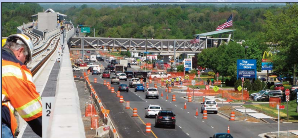
FINISHING TOUCHES: Crews work along the aerial guideway while others prepare for sidewalks along the westbound lanes of Route 7. Photo by Chuck Samuelson, Dulles Corridor Metrorail Project
