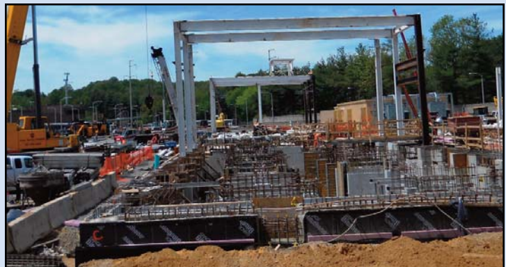
EXPANSION AT WEST FALLS CHURCH RAIL YARD: The basement floor slab for the Service and Inspection Building has been placed and the steel framing is underway. In addition the wall and pier foundation for the Long Track Sound Cover Box, designed to minimize noise, is done. Photo by Stephen Barna, Dulles Corridor Metrorail Project
