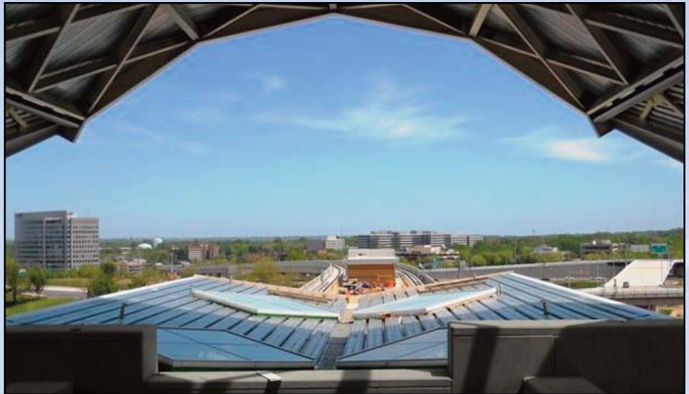
VIEW FROM THE TOP: Significant progress is taking place at the Tysons Corner Station along the northwest side of Route 123 at Tysons Boulevard. Crews continue to work on installation of elevators, the pedestrian bridges and access pavilions. Escalators are under construction; these are some of the highest escalators in Phase 1, according to construction officials. The barrel canopy, the concrete topping on the slab and skylights are almost done. Pedestrians will be able to access Tysons Corner Center via a bridge across busy Route 123. Photo by Stephen Barna, Dulles Corridor Metrorail Project
