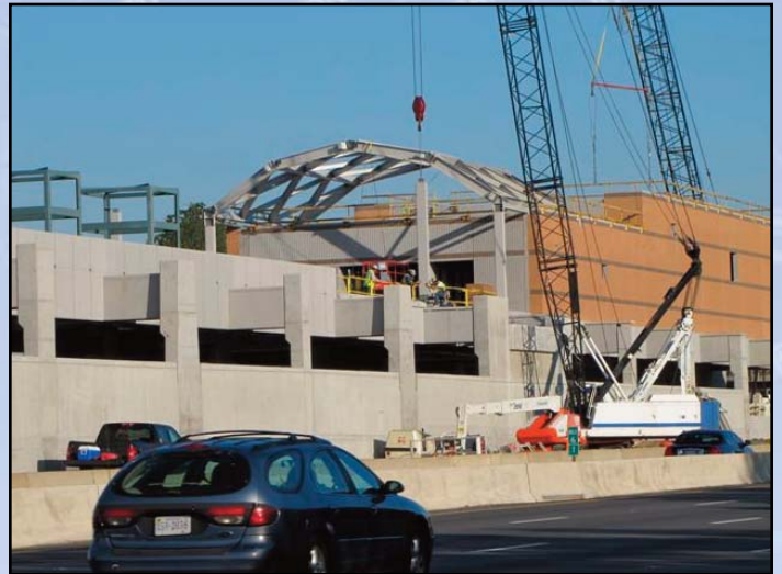
EXTREMELY VISIBLE: Construction continues on the Wiehle Avenue Metrorail Station in the median of the Dulles International Airport Access Highway/Dulles Toll Road, just west of the Wiehle Avenue overpass. Photo by Chuck Samuelson, Dulles Corridor Metrorail Project
