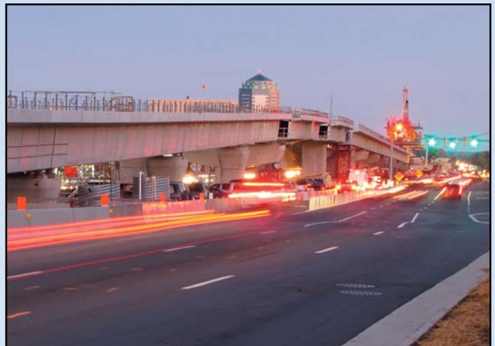
MOVING WEST ALONG ROUTE 7: Dulles Transit Partners' (DTP) crews continue to build bridges for the Dulles Corridor Metrorail Project in the median of Route 7. This photo captures construction near dusk with the Sheraton Tysons in the background. A huge bright yellow horizontal crane is being used by DTP subcontractor Rizzani, an Italian company that has done bridge-building around the world. Photo by Chuck Samuelson, Dulles Corridor Metrorail Project
