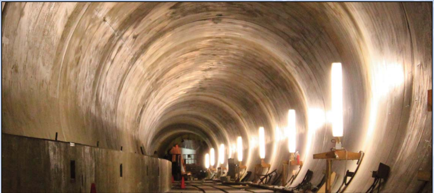
SILVER LINING CONNECTIONS: Tunnel connecting two of the four Metrorail stations in Tysons Corner take on a silvery look as work progresses. Crews will soon begin laying track here. Photo by Frank Jenkins, Dulles Transit Partners
