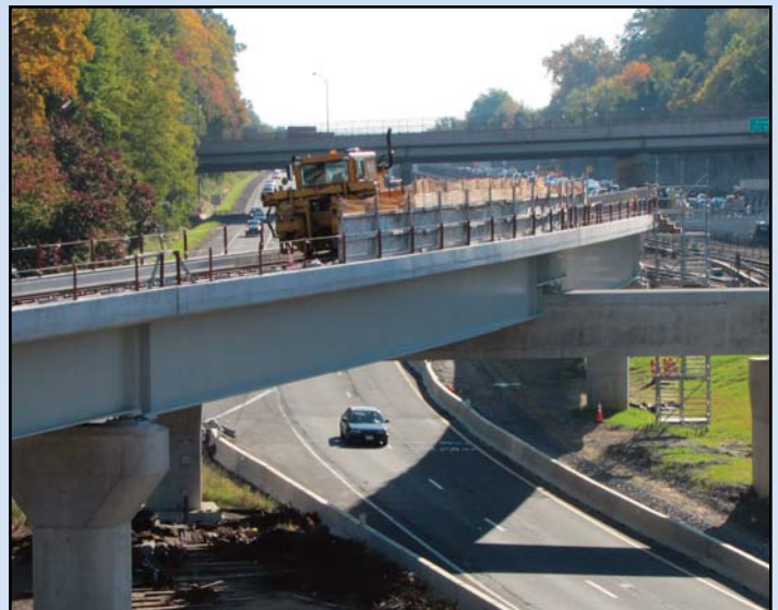
MAKING THE CONNECTION: Crews continue to fine-tune connections between the Silver Line and the existing Orange Line. Photo by Chuck Samuelson, Dulles Corridor Metrorail Project
