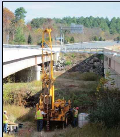
ALONG THE GREENWAY IN LOUDOUN: Capital Rail Constructors crews perform geotech work for future Phase 2 rail construction near Broad Run. Photo by Scott Evans, Dulles Corridor Metrorail Project
