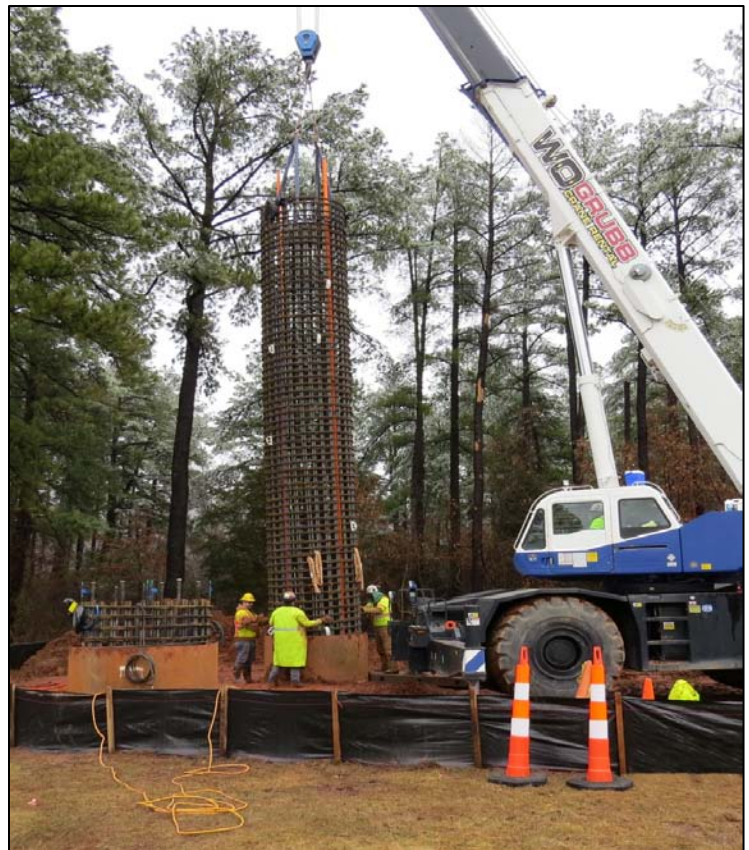
Once in the ground, concrete will be poured around these rebar cages that will reinforce the test shafts. Photo by: Chuck Samuelson, MWAA
