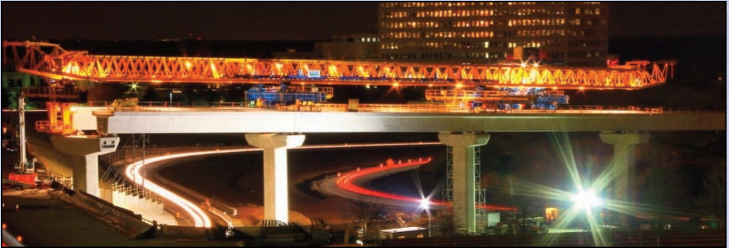
Construction of bridge spans using a giant horizontal crane continues along Route 123 near the Capital Beltway in Tysons Corner Photo by Igor Scherbakov, Dulles Transit Partners
