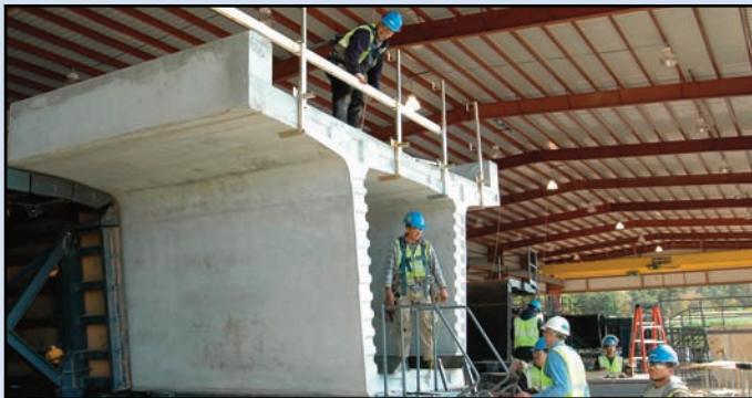
Segments are manufactured off-site at a precast facility near Dulles Airport. Photo by Dulles Corridor Metrorail Project
