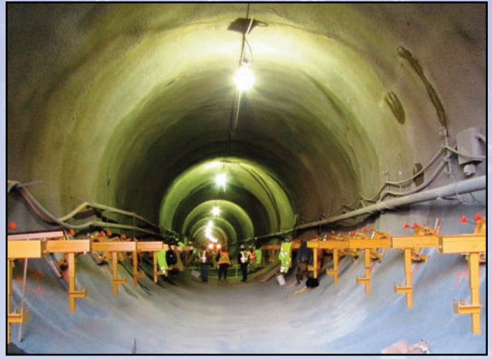
Mining for both inbound and outbound tunnels was completed last year and crews are now providing additional reinforcements.
