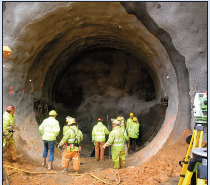
Miners feed support pipes from the Drill Jumbo's manbasket on the first day of the outbound tunnel's excavation. Photo courtesy Dulles Transit Partners
