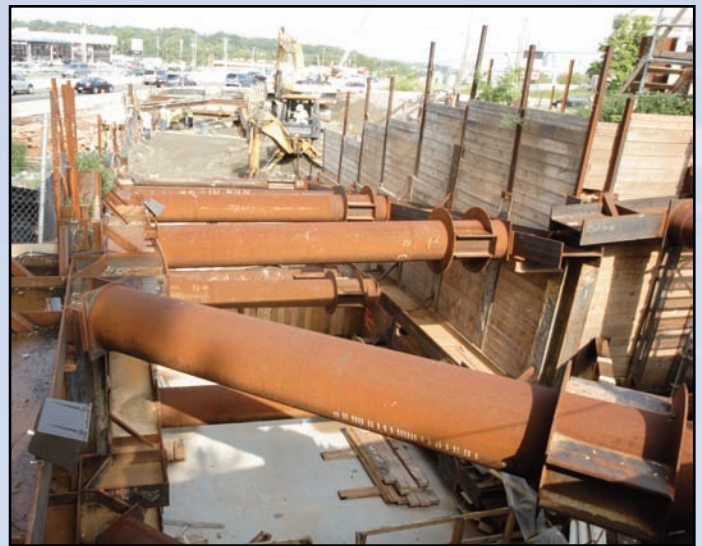
The west end of the cut and cover portion site with westbound Route 7 traffic moving in the background of this photo.
