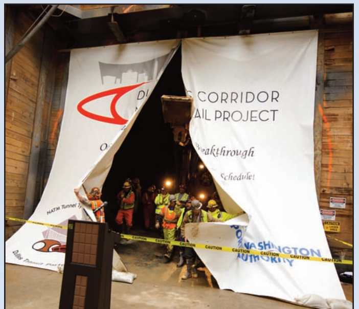
Crews for Dulles Transit Partners, the project's design-build contractor, celebrate the completion of the mining of the outbound tunnel.
