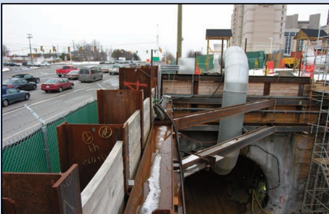
The inbound tunnel construction located directly next to the green fence along Route 123 near International Drive. Photo by Dulles Corridor Metrorail Project
